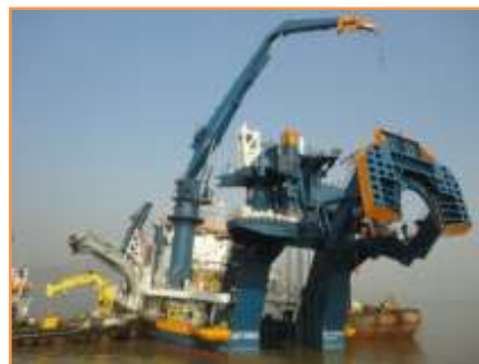
A Royal Boskalis dredger deepening the Mumbai Harbour channel –Making way for Bigger Ships!
